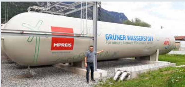
Mr. Amir Habibelahian shows the hydrogen tank of the MPREIS electrolysis plant in Völs, Austria.
