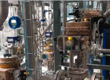
Sustainable production of hydrogen at MPREIS in Völs, Austria using SAMSON globe valves for throttling and on/off service.
